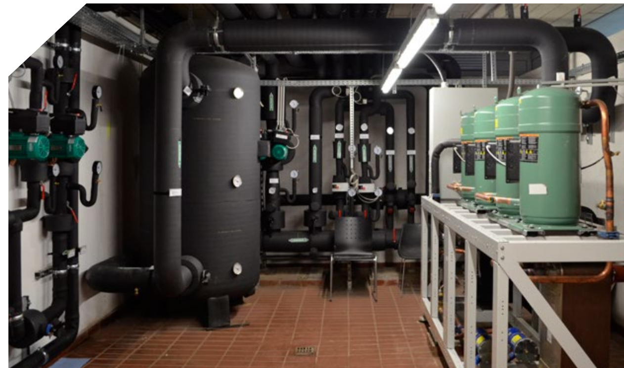
The new BITZER refrigeration system in the WIFO office building in Vienna.
